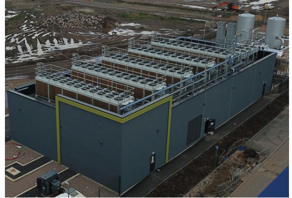
SmartParc Energy Centre, Derby Source: SmartParc
